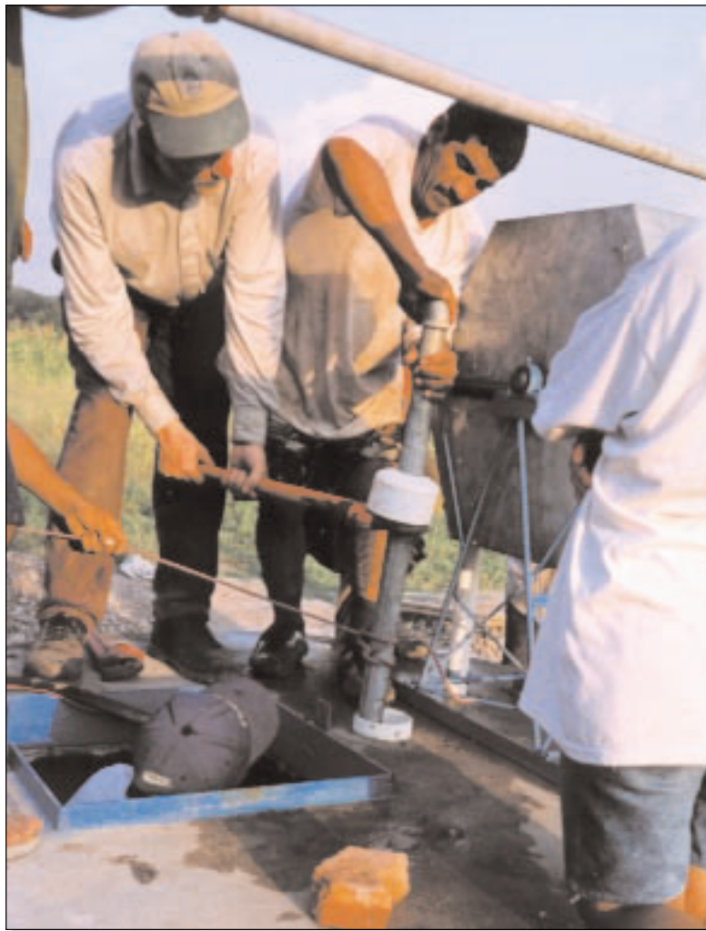
Figure 2 Technicians secure solar pump in the well
