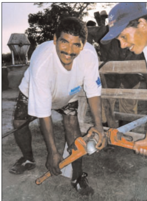
Figure 3 (Accion contra el hambre) Action Against Hunger – technician prepares pipe for solar pump installation
