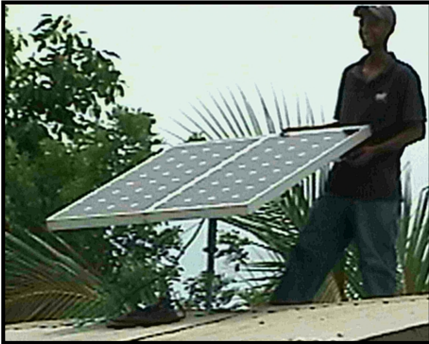
Local PV Technician installs modules on school in Batalla July 1, 2005. Batalla is located in the remote Honduran Moskitia. The project has experienced long delays due to the logistical challenges working in the region presents.
