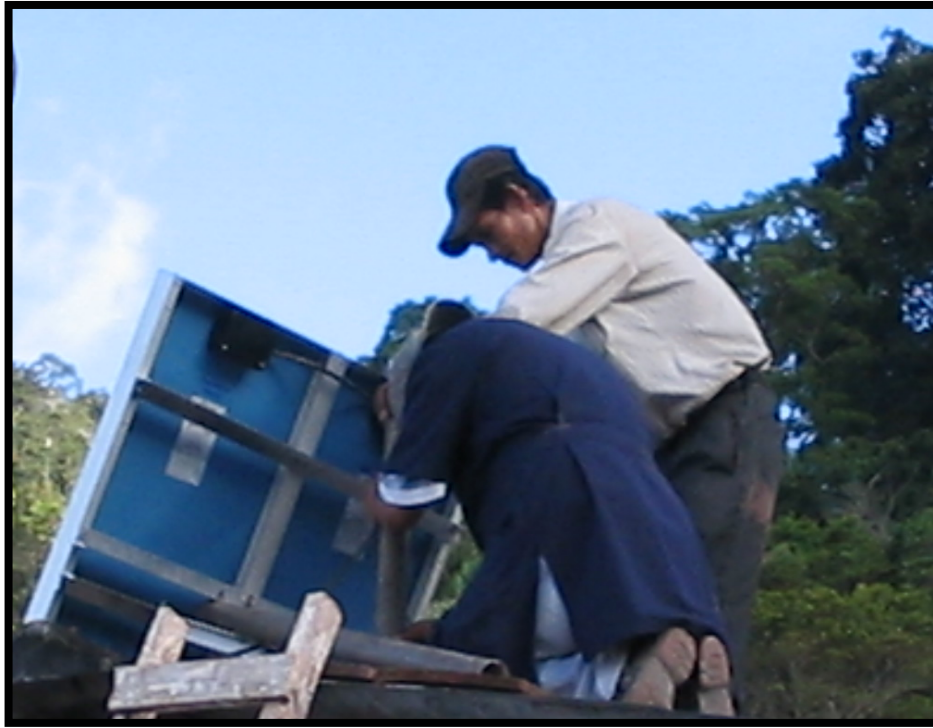
Community member assists Soluz Honduras PV Technician mount the PV array September 2004.
